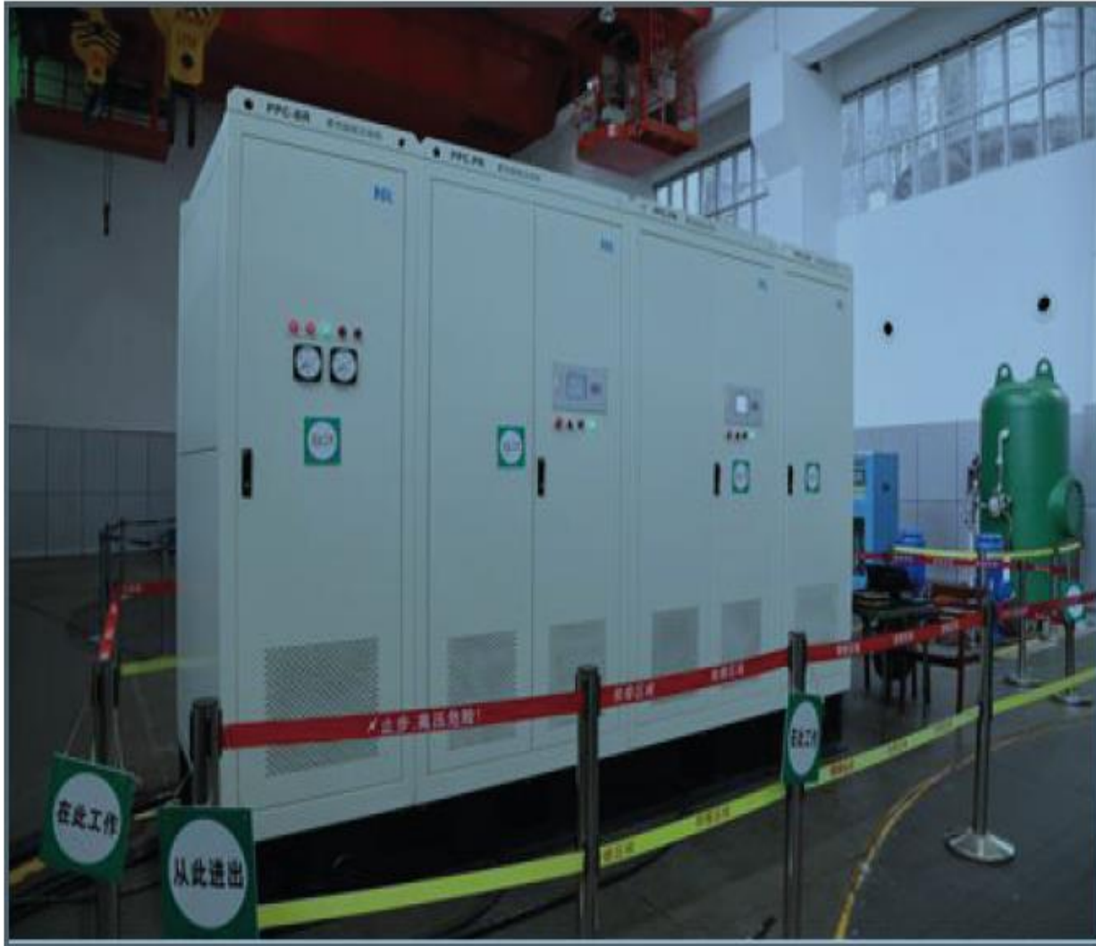
Figure. 3 Engineering prototype of flexible excitation system
