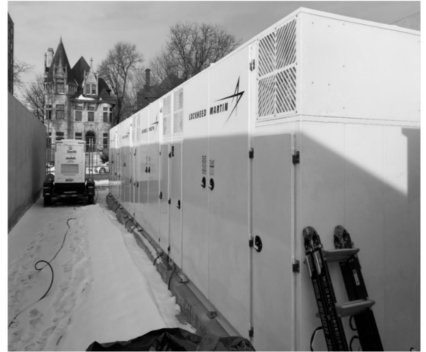
Battery Energy Storage Installation
